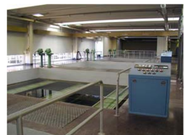
Filter beds are the final stage of water treatment.
