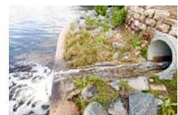
Stormwater outflow pipe
