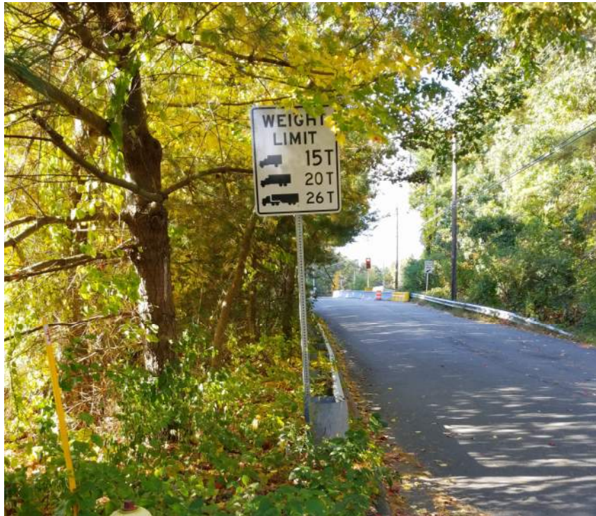
Bridge is Posted for Load Limits
