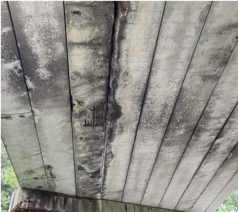
Exposed and Broken Steel Reinforcement
