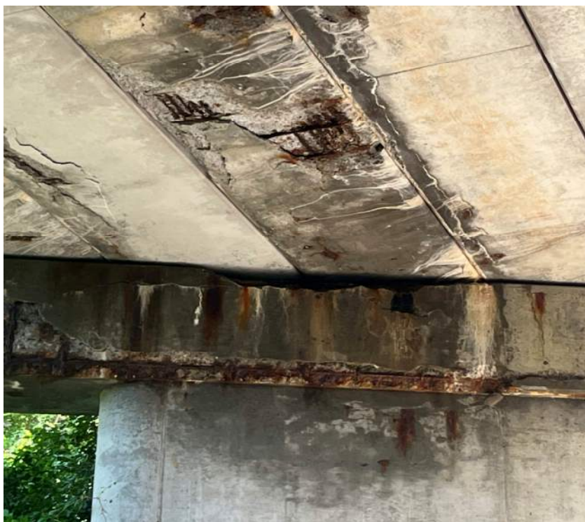
Deterioration of Pier Cap
