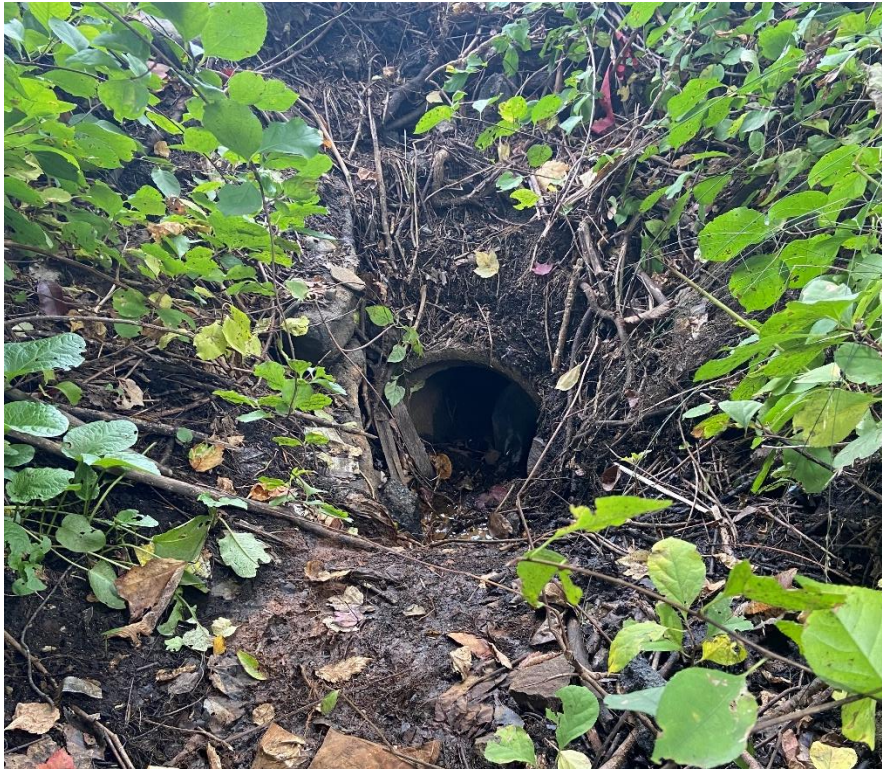
Photograph 4.2: Southeast wetland—Outfall pipe conveying storm overflow from DP-3 (taken on 9/29/2021)
