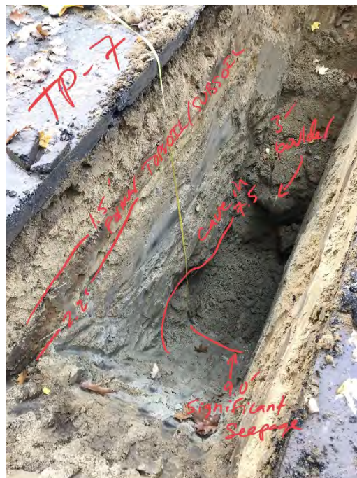
Photo 14: Test pit HA21-TP7. Water seepage noted at about 9 ft bgs. Sidewall of test pit collapsed at approximately 7.5 ft bgs. A 3 ft diameter boulder is noted within the Glacial Till layer.
