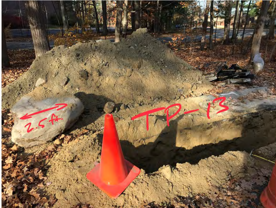
Photo 23: Stockpile of soil excavated from test pit HA21-TP13. Encountered a 2.5 ft diameter boulder during the excavation.
