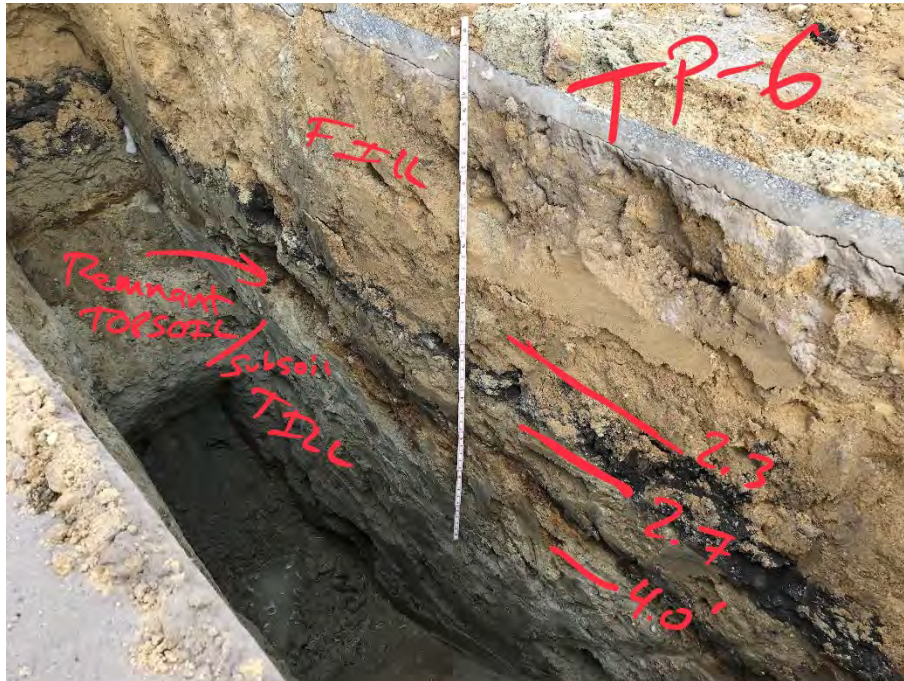
Photo 13: Sidewall of test pit HA21-TP6 depicting soil stratigraphy. Top of Glacial Till is approximately 4 ft bgs and is underlying an approximately 1.7 ft thick layer of former/remnant Topsoil/Subsoil. Water is visible at the bottom of the excavation.
