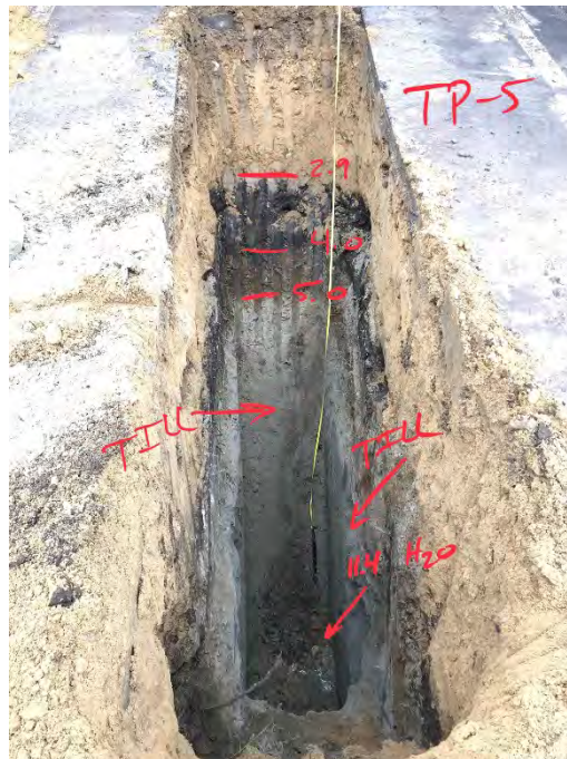
Photo 10: Glacial Till encountered at approximately 5 ft below a 2.1 ft thick layer of former/remnant Topsoil/Subsoil in test pit HA21-TP5. Water seepage and cave-in observed at the bottom of excavation at about 11.4 ft bgs.
