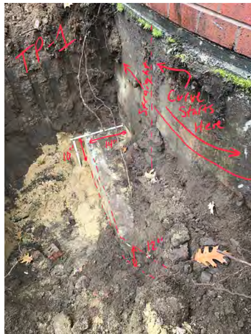
Photo 2: Photo of existing strip footing encountered at test pit HA21-TP1. Top of footing encountered 42 in. bgs. Footing was determined to be 10 to 12 in. thick. The footing protruded beyond the face of the foundation wall by 14 to 16 in.
