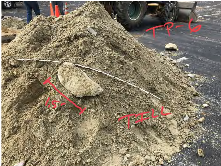
Photo 12: Stockpile of Glacial Till excavated from test pit HA21-TP6. Encountered a 1.5 ft long boulder in the Glacial Till.
