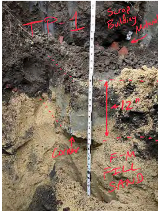
Photo 3: Corner of existing footing foundation encountered in test pit HA21-TP1. Imported Fill (sand) was encountered below the bottom of the footing and above the naturally deposited glacial soils.
