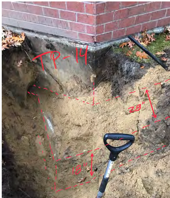
Photo 24: Existing footing foundation encountered in test pit HA21-TP14. Top of footing encountered at 42 in. bgs. Footing was determined to protrude beyond the exterior face of the foundation wall by 28 in. where measured parallel to the wall. The depth of the footing was determined to be 18 in.
