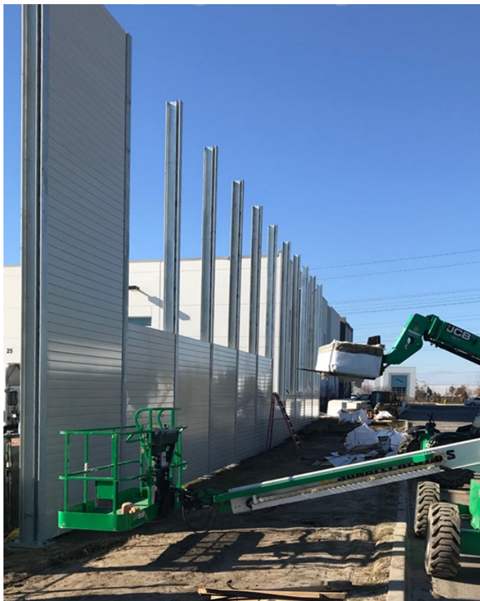
Example 2: Sound wall under construction showing I-beams installed on footings with noise barrier slats being installed
