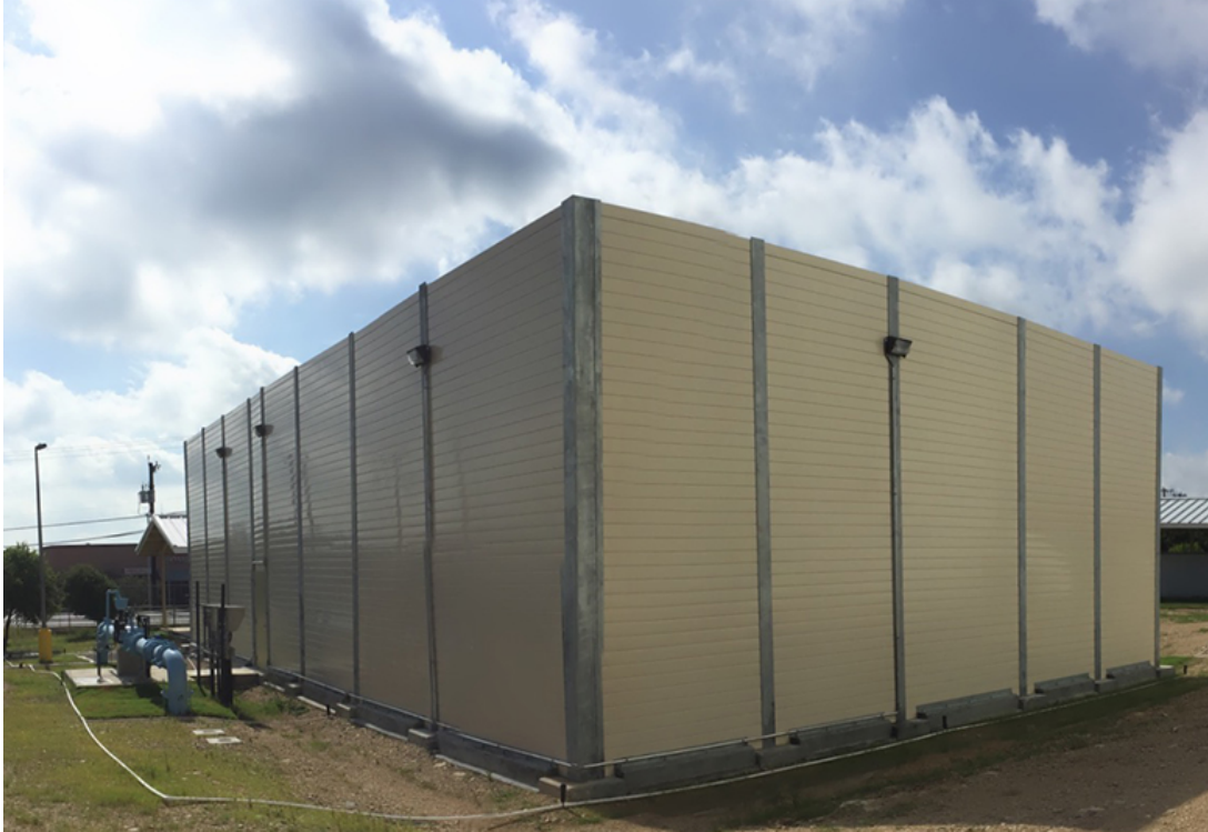
Example 1: Sound wall surrounding equipment. Please note, the Battery Energy Storage project does not propose to include exterior lighting
