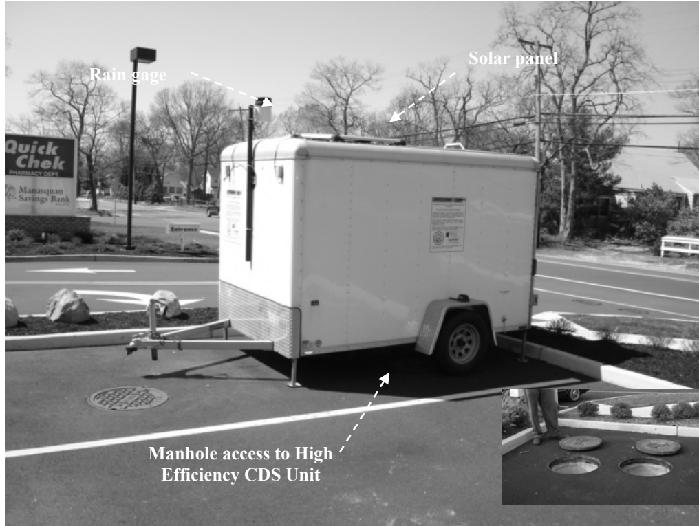
Figure 7 View of Mobile Monitoring Unit (MMU) installed at the Manasquan Savings Bank study site
