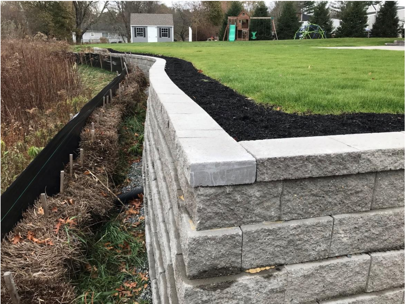
Picture 4. Staked-in hay bales and silt fence at the limit of work between a retaining wall/landscaping project and a wetland in the backyard of a single-family home in Andover.
