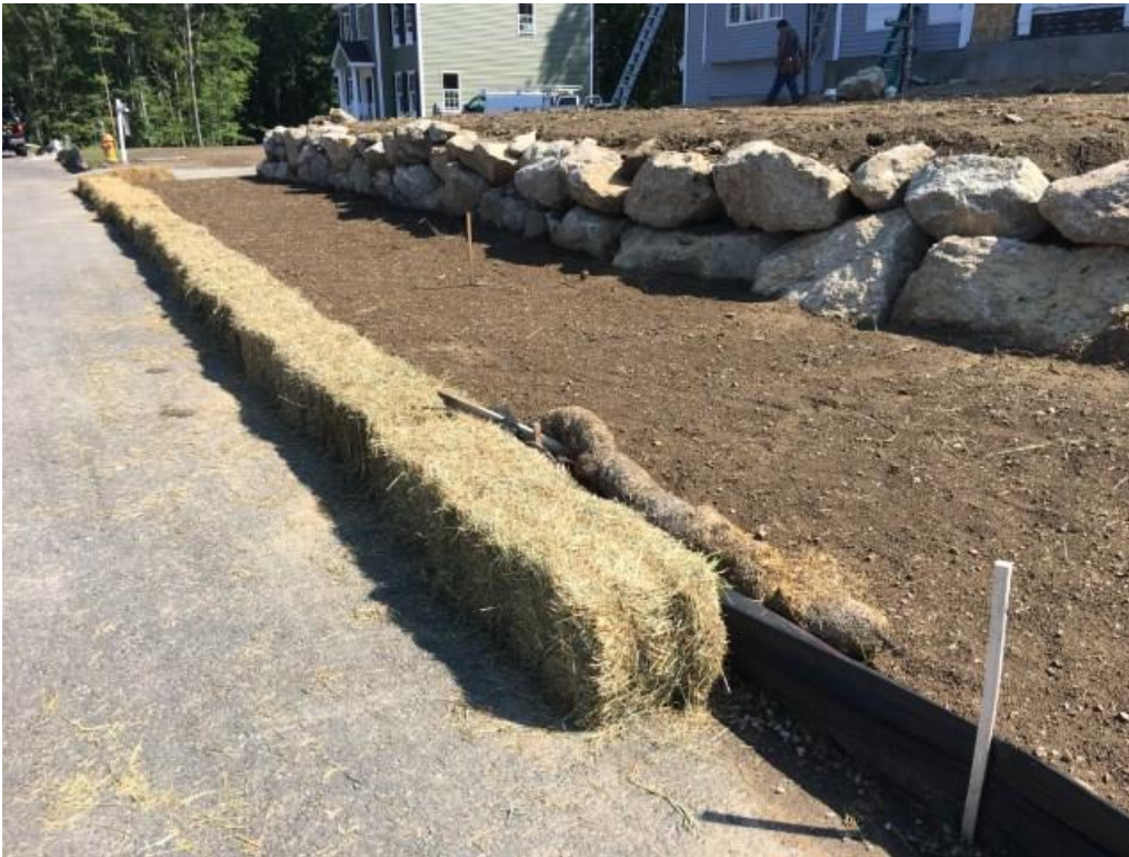
Picture 12. Straw wattles, hay bales, and silt fence placed between a newly graded house lot and the roadway in Andover. Prior to hydroseeding, soils are disturbed. This soil is highly vulnerable to being washed away during a rain event.
