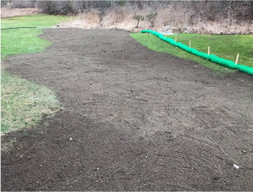
Picture 5. Staked in mulch sock at the limit of work between a landscaping project and a wetland in the backyard of a single-family home in Andover.
