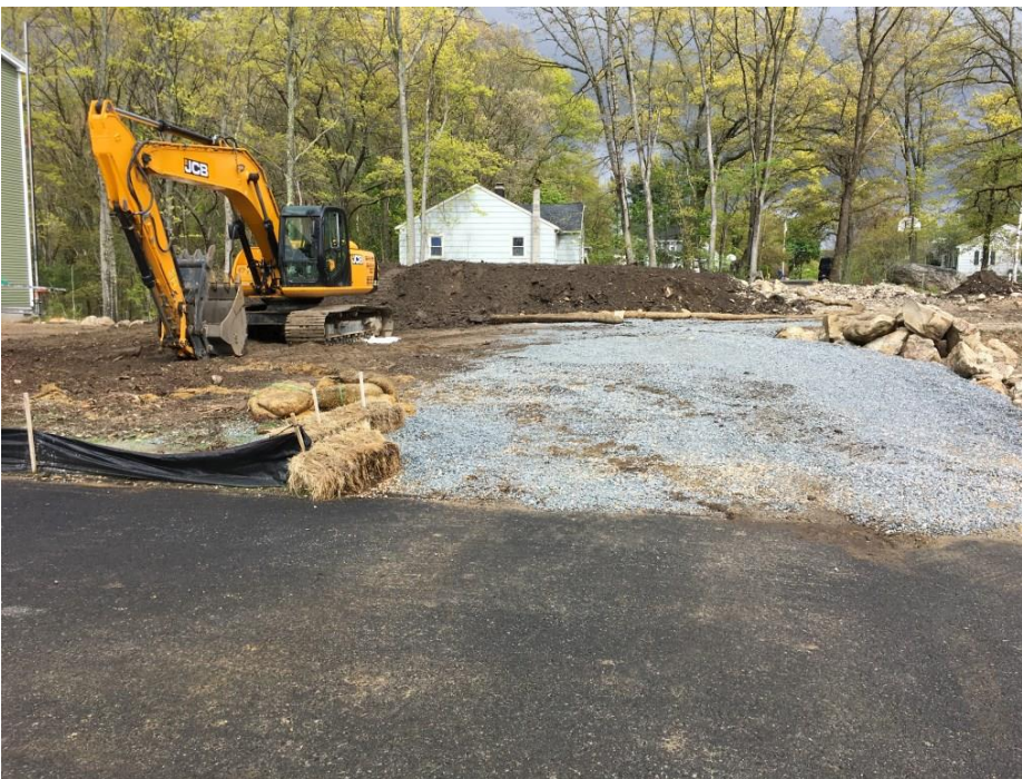
Picture 10. Crushed stone in place at the entrance to a construction site in Andover.
