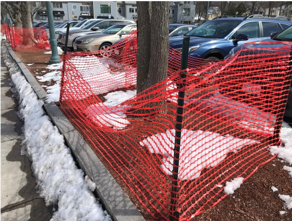
Picture 8. Staked in snow fence protecting street trees in an active construction site in Andover. Street trees to remain.
