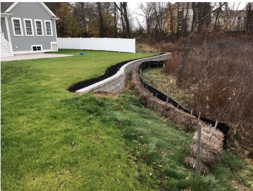
Picture 6. Staked-in hay bales and silt fence at the limit of work between a retaining wall/landscaping project and a wetland in the backyard of a single-family home in Andover.
