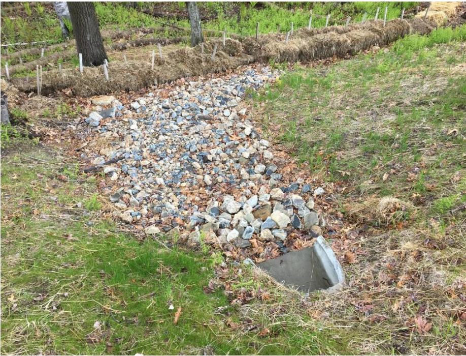
Picture 9. Crushed stone/rip rap at the outlet of a stormwater infiltration basin in Andover.
