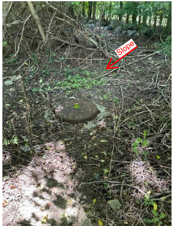
Manhole in the swale with the P/L stone wall on the right and the retaining on the left.
