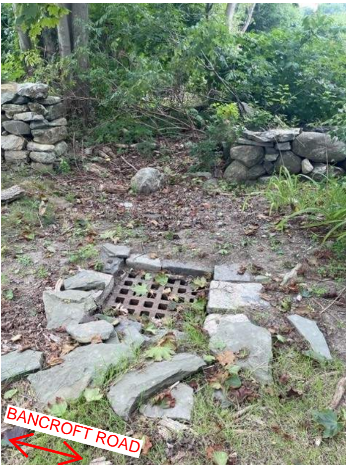
Catch Basin along Bancroft Rd. just East of the entrance & connected to the drainage system.
