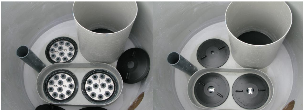
Figure 7 Top view photos of the Jellyfish Filter JF4-2-1 deck with two hi-flo cartridges and one draindown cartridge installed with cartridge lids off (upper left image) and cartridge lids on (upper right image). The backwash pool weir encloses the hi-flo cartridge. Also shown are the maintenance access pipe (large), pressure relief pipe (small), and the outlet opening (lower right in each image).
