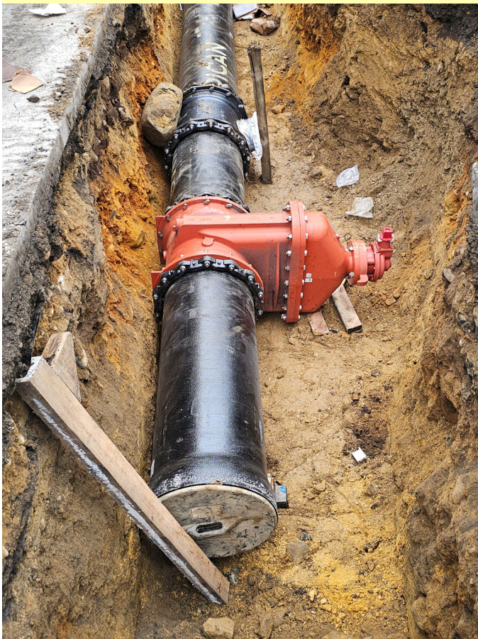
A 20" gate valve and hydrant tee installed on the new transmission main on Argilla Road.
