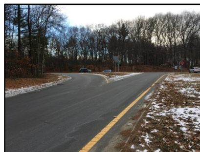
Image 5: Lack of YIELD signage and markings on Dascomb Road channelized lane.
