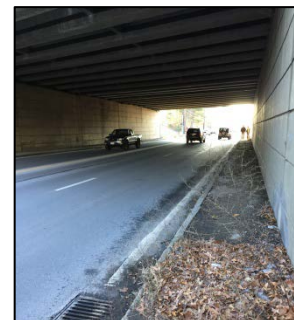
Image 3: Debris located on sidewalk below I-93 overpass.
