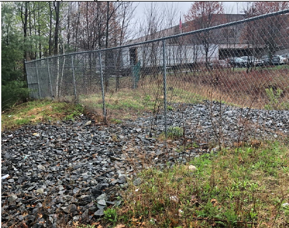
Figure 4 – infiltration basin overflow in good condition, basin does not appear to be overflowing as rip rap appears to be in untouched condition
