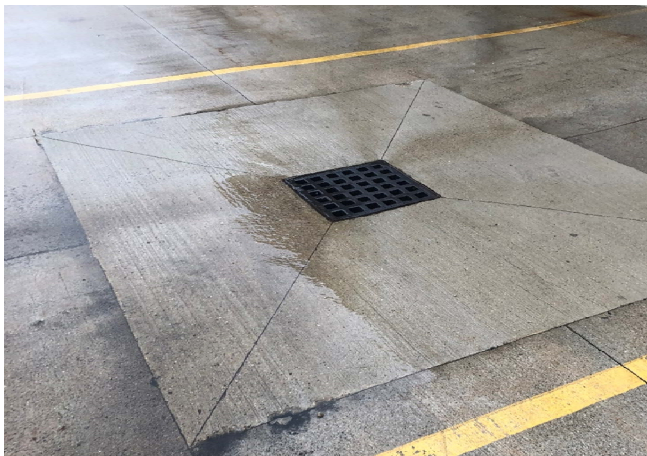
Figure 1 – catch basin, appears to have been swept recently, water flowing freely, no sedimentation visible
