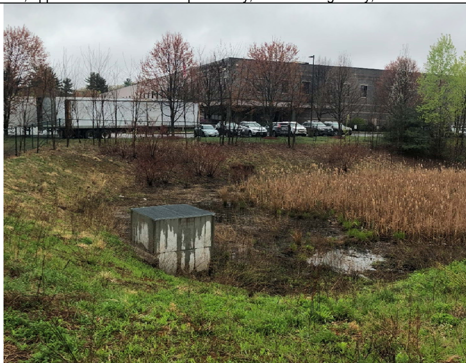
Figure 2 – infiltration basin with negligible standing water, after receiving 2"+ rain over 7 day span
